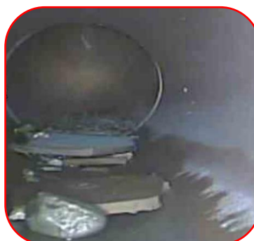
Example of a Debris Found
