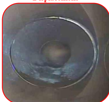
Example of a Joint Displacement
